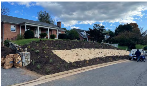
Jute netting on a slope planting in progress. After planting, the jute is hidden under mulch, where it biodegrades over time. Photo credit: Pete Corbino, District Native Plants.
