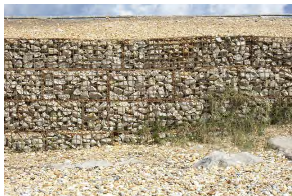
A gabion wall on the English Channel near Bournemouth, shoring up the ends of an Iron Age settlement. Photo credit: Mr. Ignavy, geograph.uk.org .
